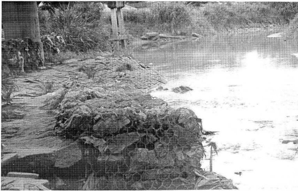
Figure 6 : Use of Gabions as a Temporary Scour Countermeasure at Plentong River Bridge (looking downstream)
